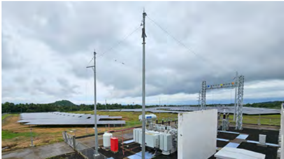
The substation facility at CARE.
