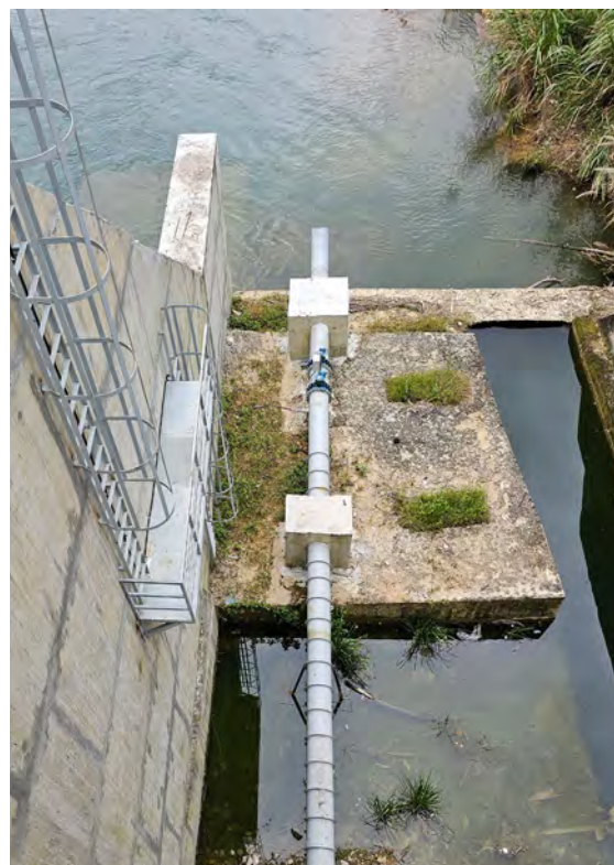
eFlow monitoring system in place at SG1 plant.
